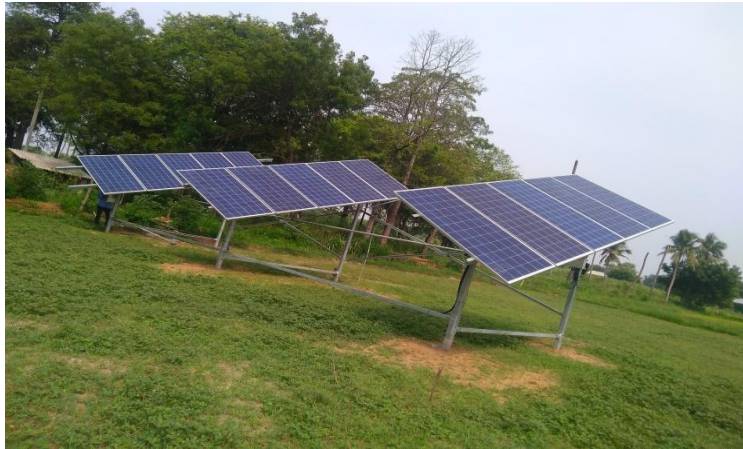
Plate.1 Solar PV water pumping system at central farm
